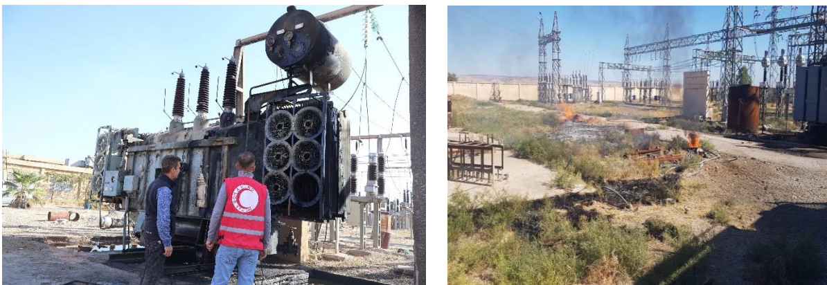
Electricity stations in Qamishli and Tirbespiye (Images by KRC Media Office)
