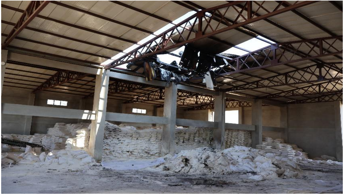
Damaged grain and flour storage facility in Qamishli (Image by KRC Media Office)
